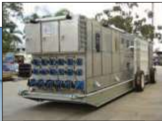
Mobile mining substation and switchgear
