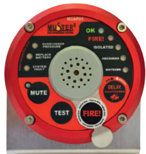
Muster II Alarm Panel
